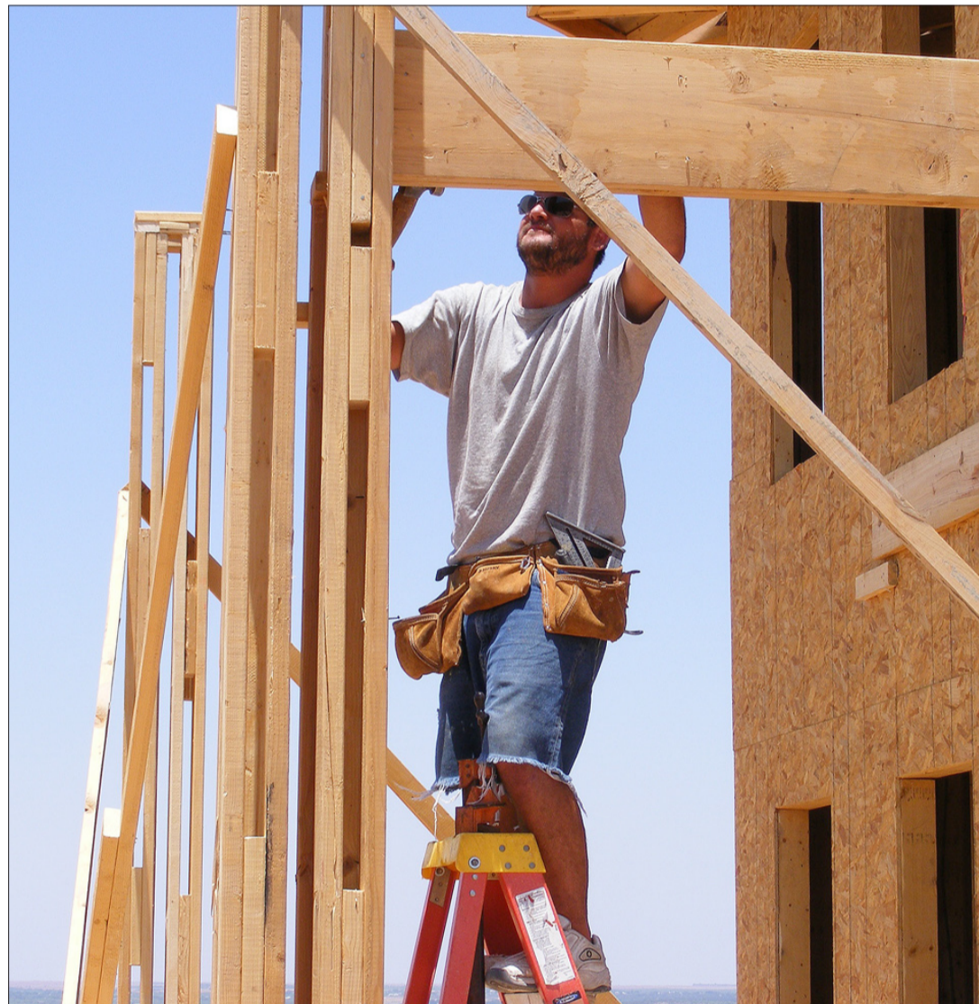
Heath Moncada works on the new Sharp Imaging building on South Highway 87 Tuesday afternoon. The building should be completed in January, officials said.
