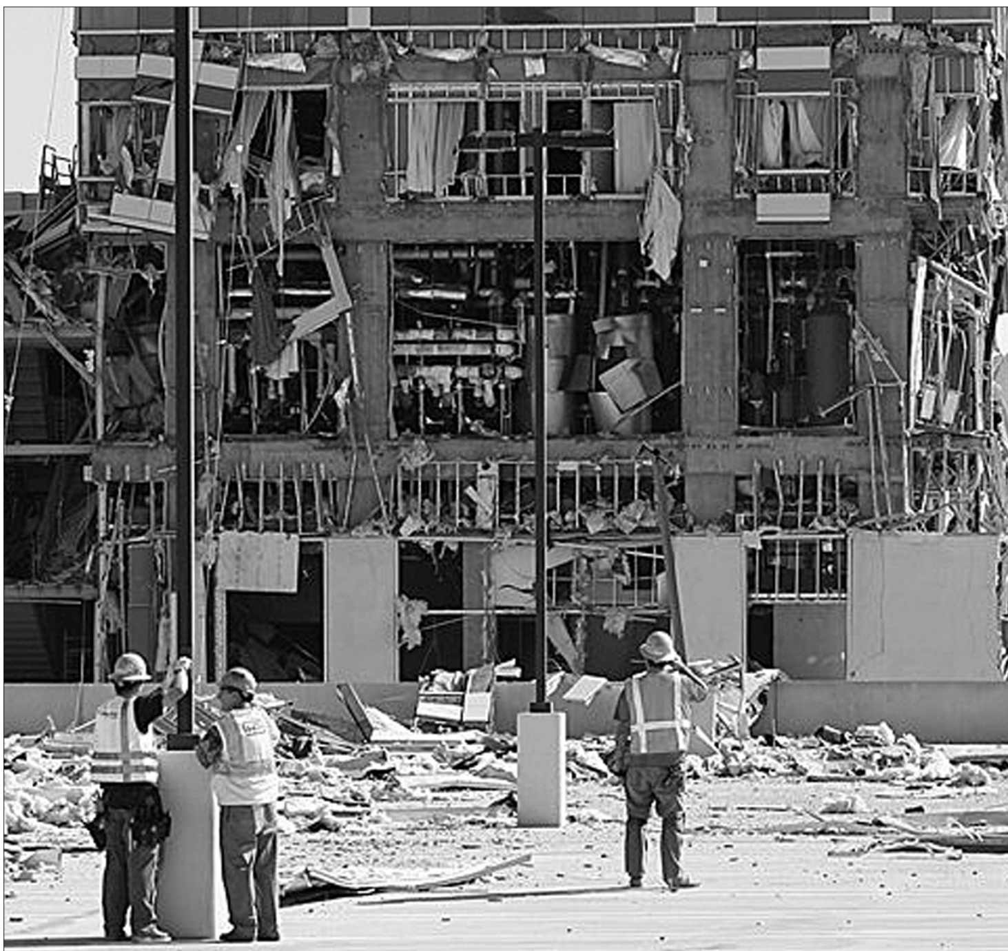
Workers stand in debris in front of the blast area of a section under construction at the Hilton Hotel where an explosion ripped through the floors Monday in San Diego. The explosion, which was felt throughout downtown, rocked the hotel under construction and 13 workers were injured, five critically, authorities said.
