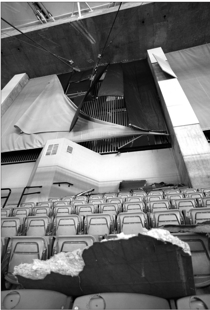
AP photo/Dave Martin Debris lies in the seats of the upper section of the Georgia Dome after a severe storm blew in several sections of the wall above, dropping debris into the seats and damaging the facility and surrounding buildings. The storm caused a delay in the Alabama-Mississippi State basketball game during the Southeastern Conference basketball tournament in the Georgia Dome in Atlanta Friday.
