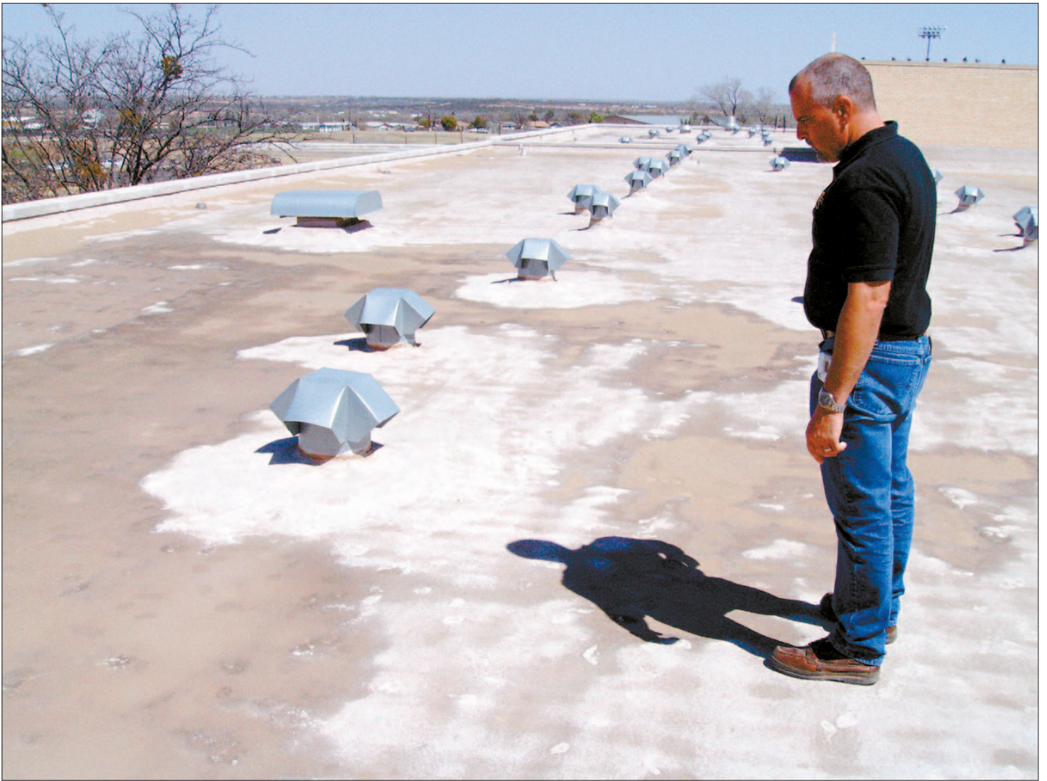
Wayland Pierce, director of transportation and maintenance for Big Spring Independent School District, inspects the roof at Big Spring High School Friday. The darker-colored portions of the roof indicate water seepage under the foam covering. Voters will decide on May 10 whether to approve up to $2.8 million to repair the structure.
