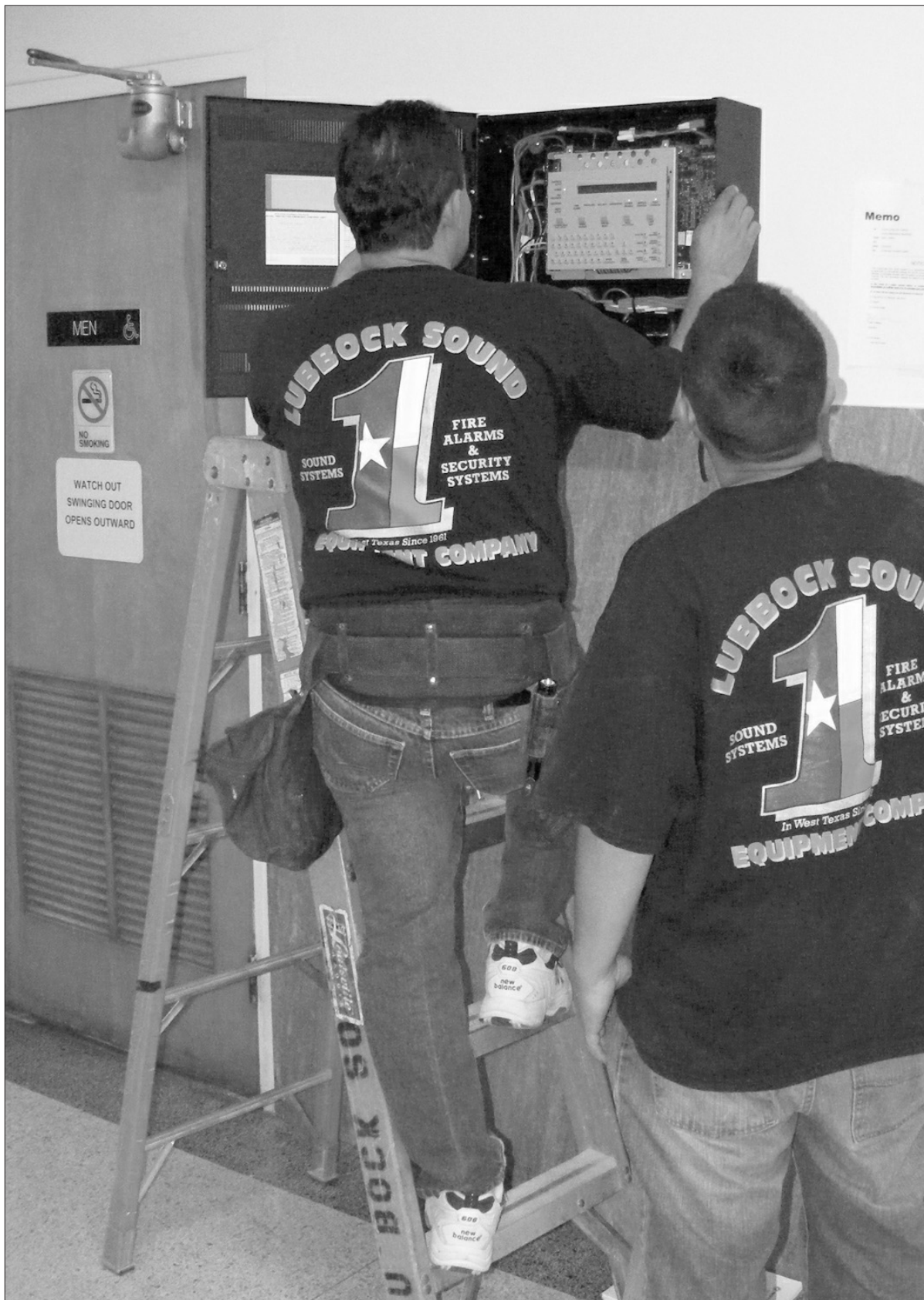
Workers make some last minute adjustments to a jail fire alarm system at the Howard County Courthouse May 21. The jail, closed by state order for six months, was allowed to reopen in May after passing life safety standard tests.
