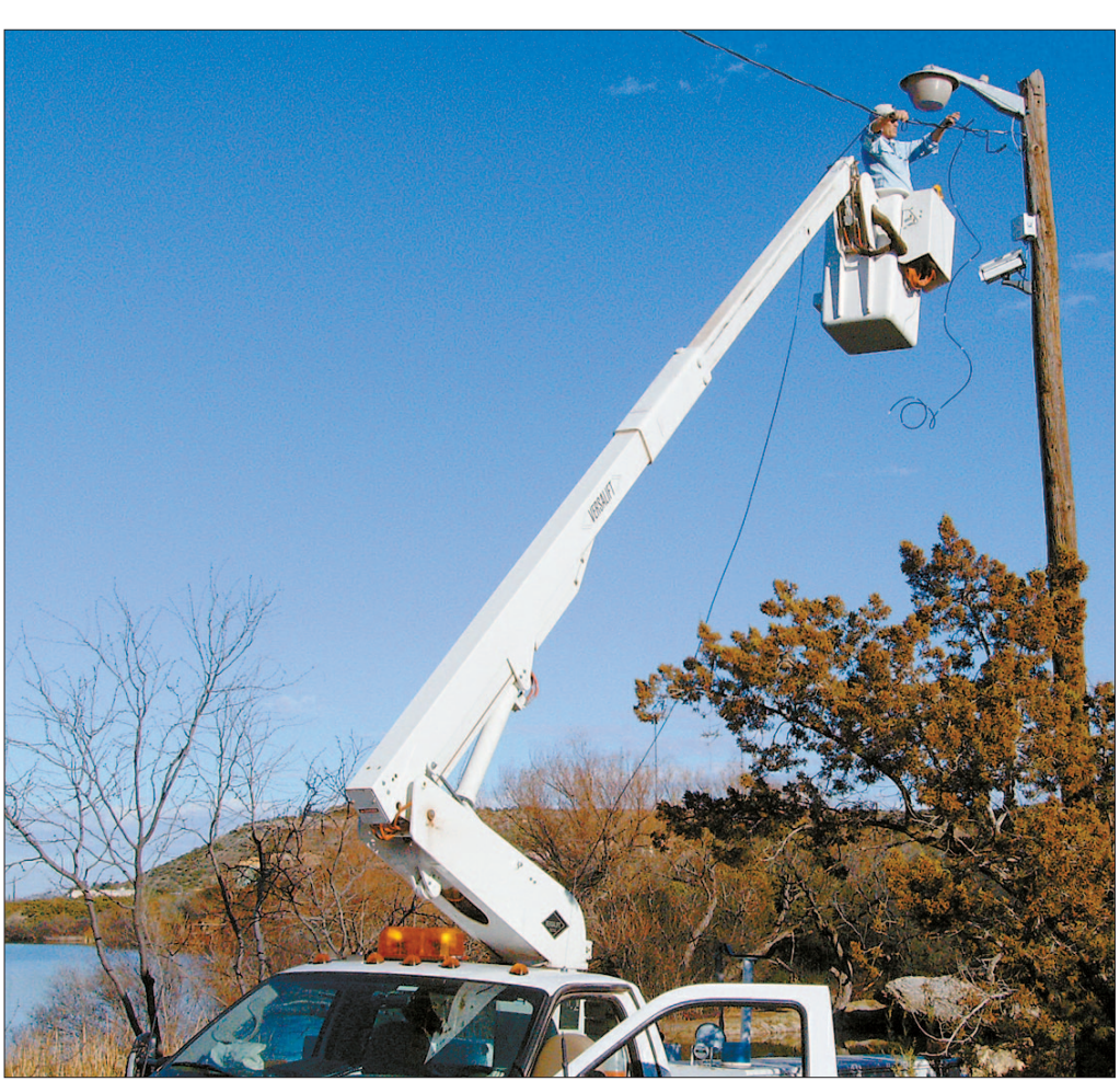
Work crews were busy at the Big Spring Tuesday, installing a trio of security cameras which officials hope will help combat vandalism and other criminal activity at the historic site.
