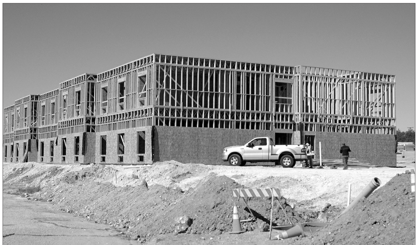
Work continues on the new Best Western motel, located on the north side of Big Spring on U.S. Highway 87, Friday afternoon.
