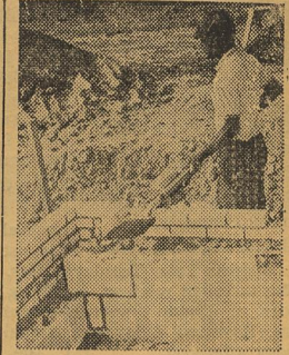
WORKER FILLS the hollow cores of wall blocks with sand to provide added shielding mass against radiation—one of several techniques used to build low-cost fallout protection into a new church at McLean, Va.
