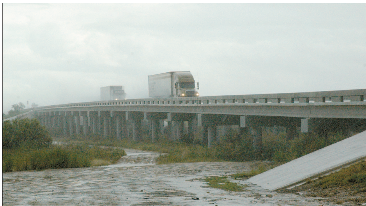
HERALD photo/Thomas Jenkins Motorists make their way across this bridge, located in northwest Big Spring on Interstate Highway 20. Local TxDOT officials say Texas bridges are inspected annually to prevent tragedies similar to the one in Minnesota that has already claimed five lives.
