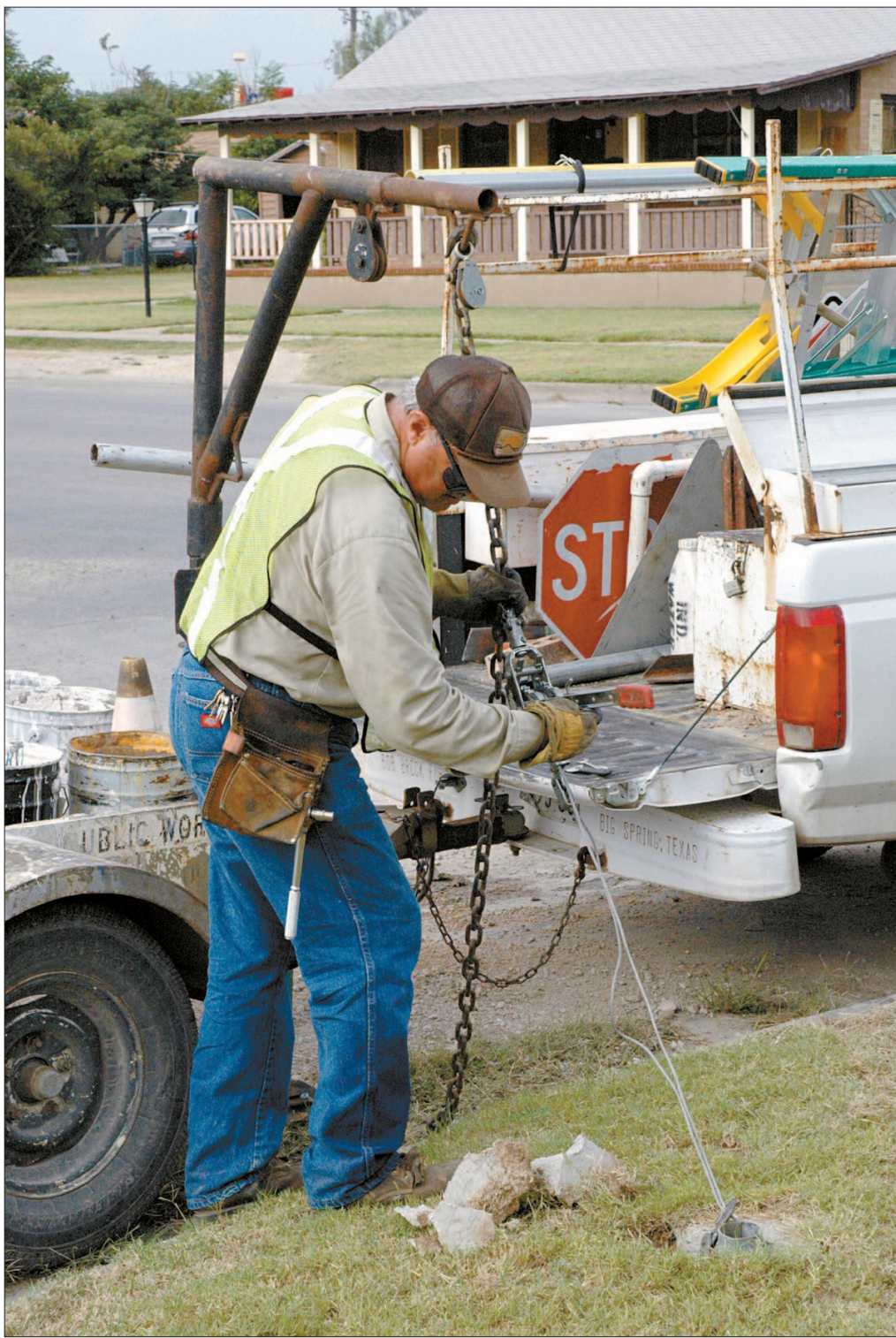
Neil Anderson, a street technician with the city of Big Spring, works to remove the base of a stop sign that was recently hit by a vehicle at the corner of 17th Street and Scurry. Anderson has been with the city streets department for more than 20 years.
