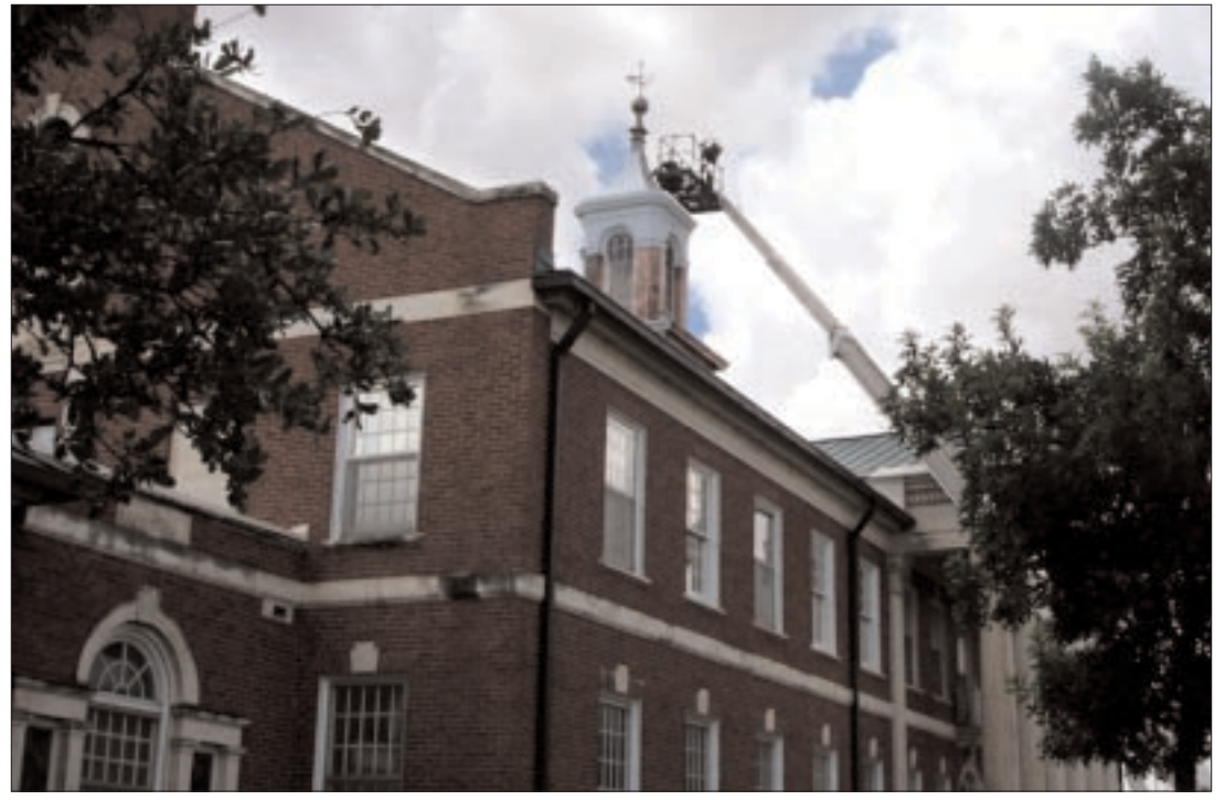
Courtesy photo Workers are shown doing renovation work on the cupola atop the administration building at Big Spring State Hospital.
