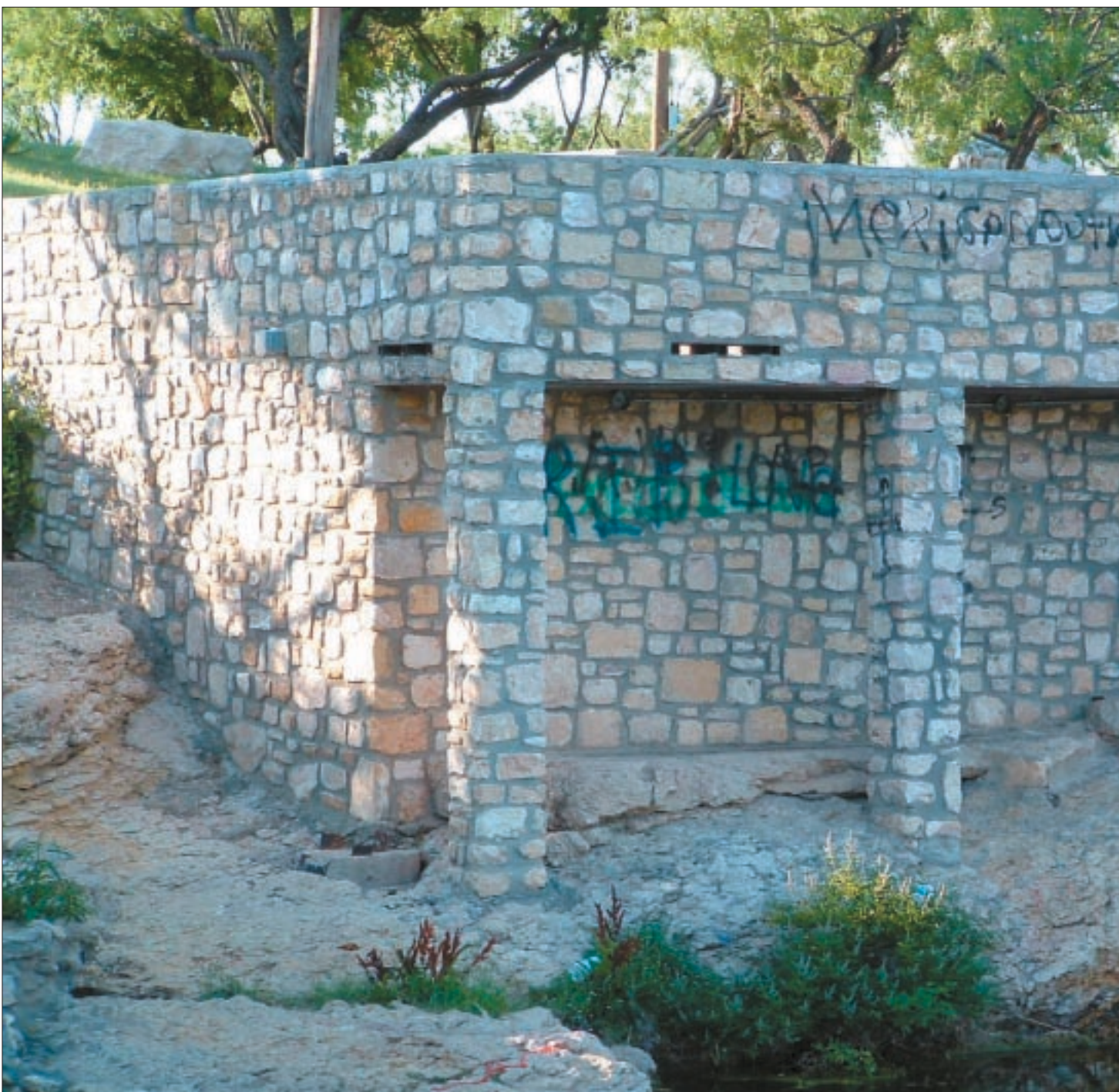
Graffiti similar to this was recently found at the historic spring in Comanche Trail Park and is expected to cost thousands of dollars to repair, according to city officials. The city of Big Spring is currently looking at surveillance equipment to protect the local landmark from future attacks by vandals.
