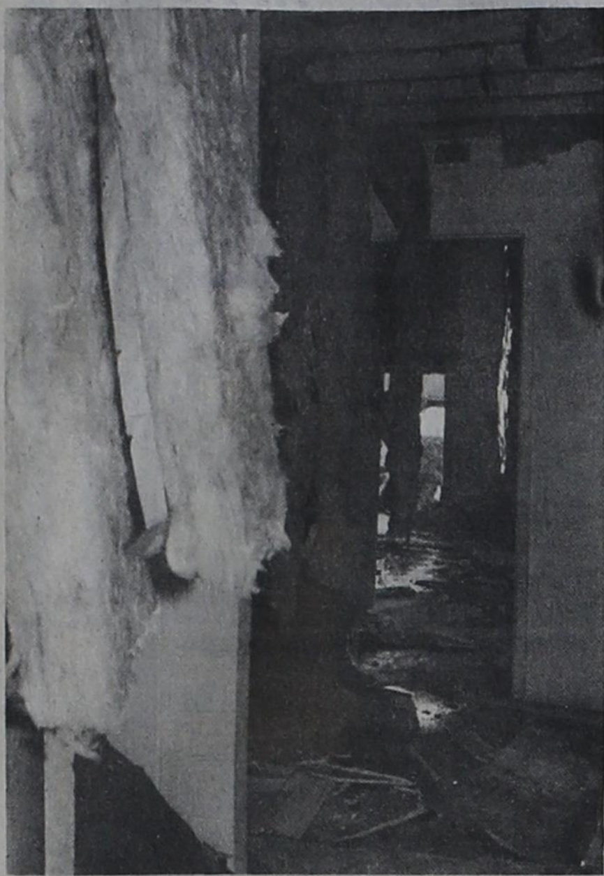
RENOVATIONS to change pre-existing efficiency apartments into two-bedroom apartments include the removal of some of the old insulation of the structure. When completed, the former 199 apartments will be reduced to 138.
