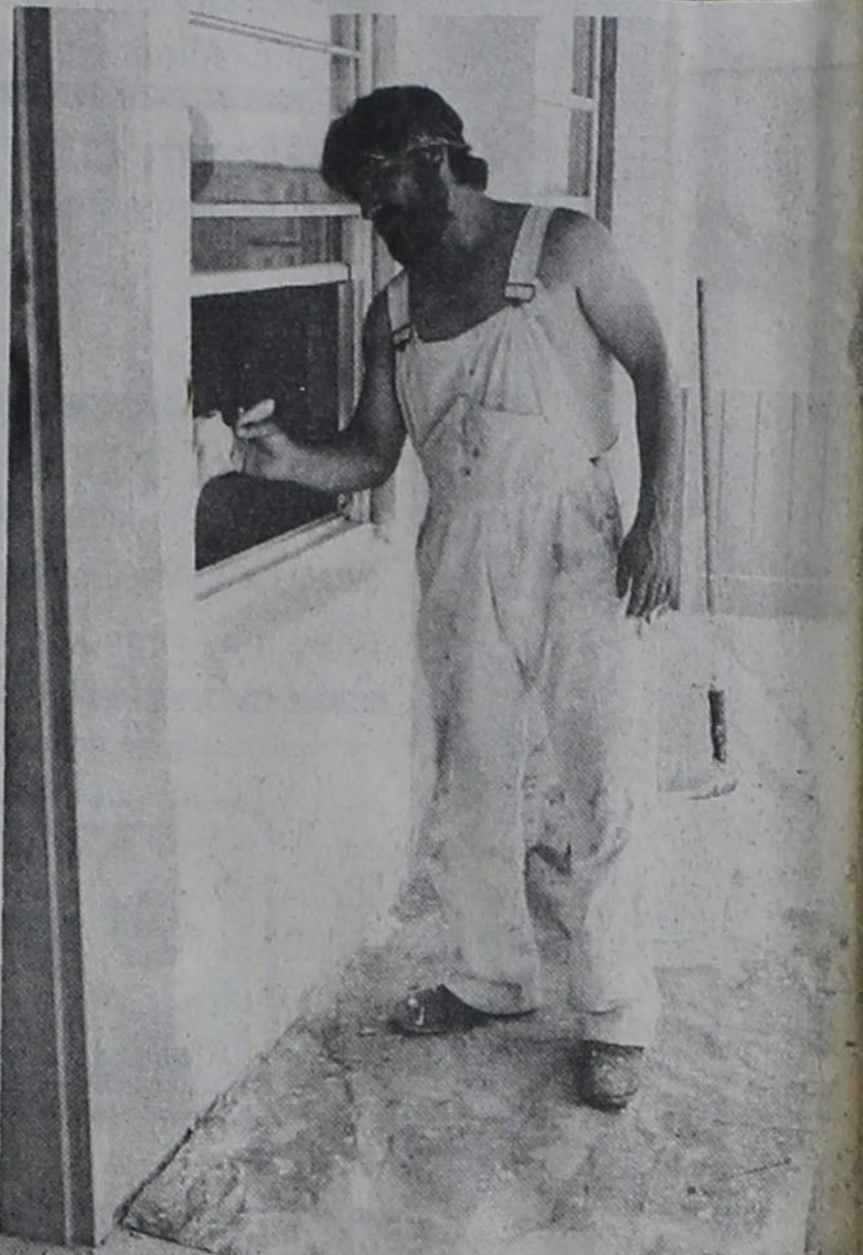
PAINTING, REMODELING and re-roofing are among the renovations scheduled to take place at the Azteca Complex. Lupe Olivarez is one of the painters working on the renovations, which are scheduled to be completed in December 1983.
