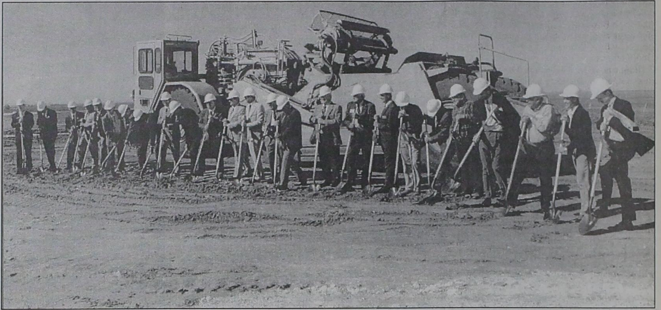
GROUND IS BROKEN by the board of directors of Golden Spread Electric Cooperative, representatives of bankers CoBank and Societe Generale, and by Yoakum County Judge Dallas Brewer and Denver City City
