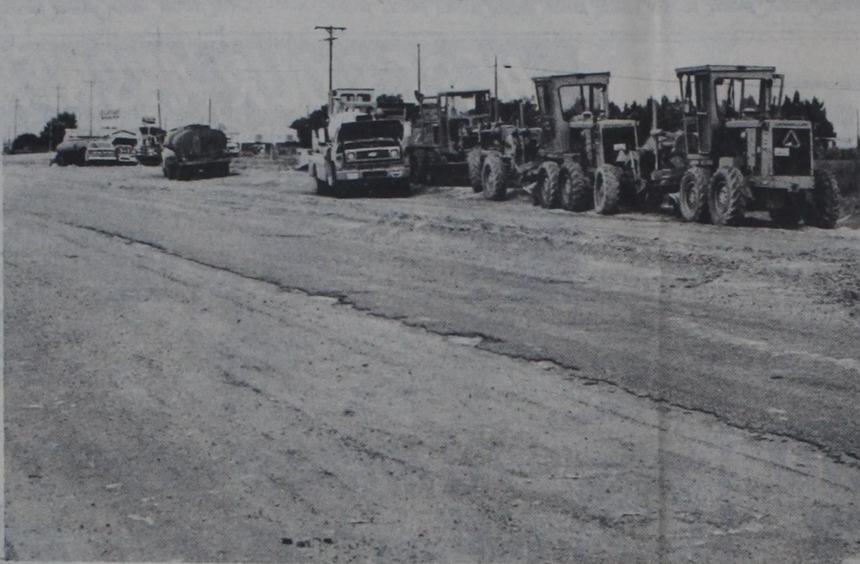
HAZARDS AND HEADACHES caused by the road construction between Nazareth and Dimmitt should be over by November, according to Rhea Bradley of the Texas Dept. of Transportation. The first layer of asphalt should be laid by then, he said. The final "riding surface" is scheduled to be put down next May.
