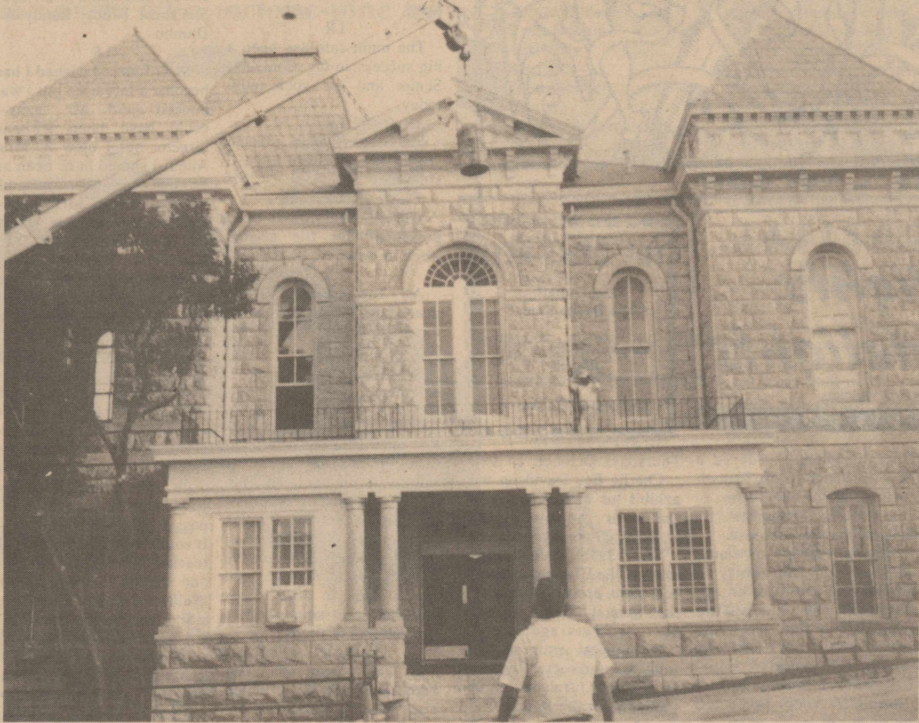
BICENTENNIAL PROJECT NEARS COMPLETION - The painting of the courthouse exterior trim was the final job in finishing up the Bicentennial Steering Committee's permanent project for the county. Courthouse and park grounds were landscaped earlier in the year, and a crew of San Angelo painters made short work of painting the trim.
