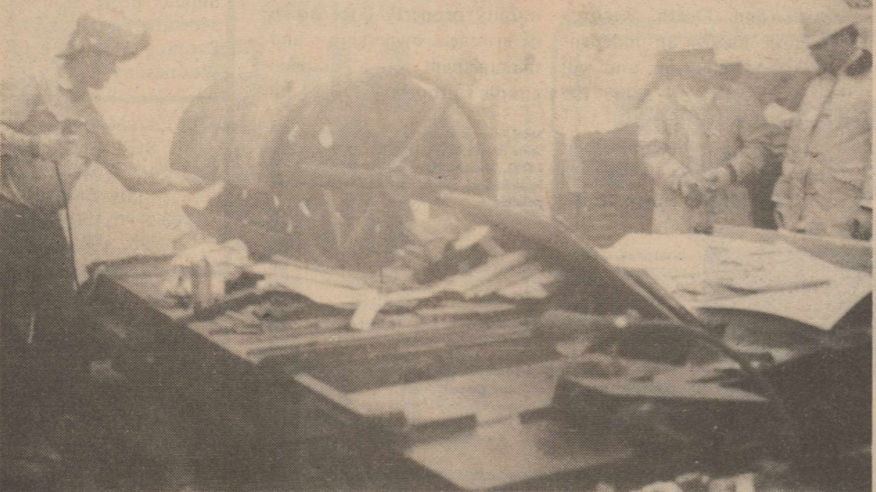
A LITTLE FIRE AND A LOT OF SMOKE and the ancient flat-bed press, which stood for the life of The Stockman at the back of the press room, was reduced to scrap metal last Thursday afternoon. Tite Bishop, demolition expert, pauses for examination during the surgery, while firemen Steve Kenley and Bob Falkner stand by for action.
