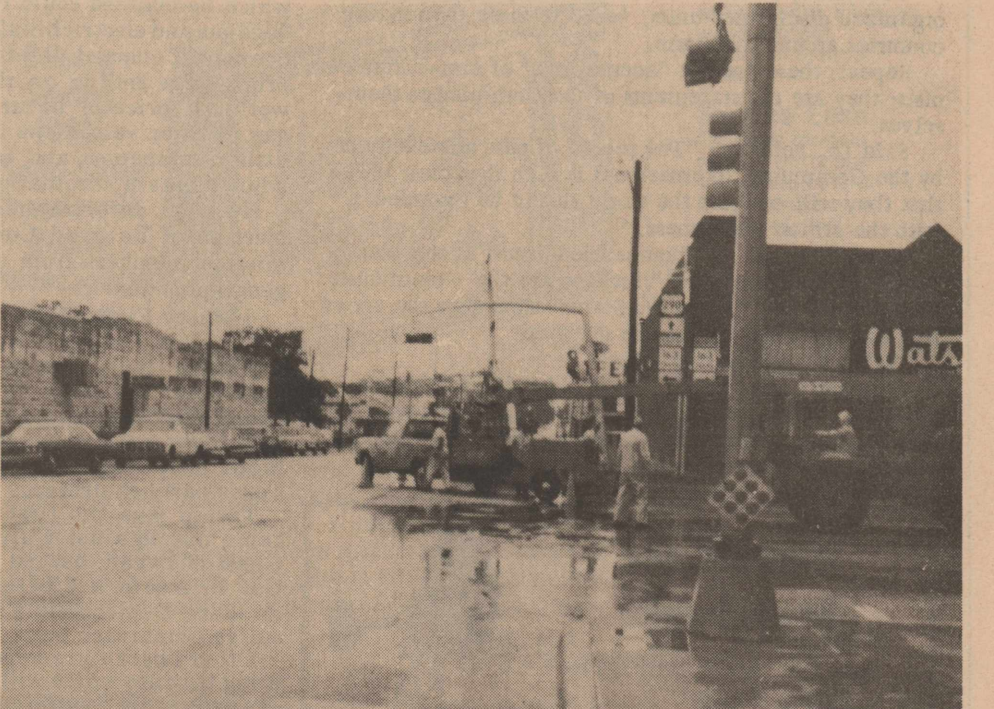
STATE HIGHWAY WORKMEN find that rain caps and coats are necessary as they arrive at a traffic light pole which was knocked over during the night, probably by a truck carrying a heavy load. The iron railing around the pole has been demolished several times by vehicles cutting the corner too short. This is a first for the heavy pole which is solidly set in concrete.
