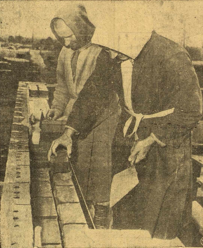
Two of the 13 ex-combat servicemen who have entered the Trappist Monastery in Conyers, Ga., lay bricks as they work on construction of a new abbey.
