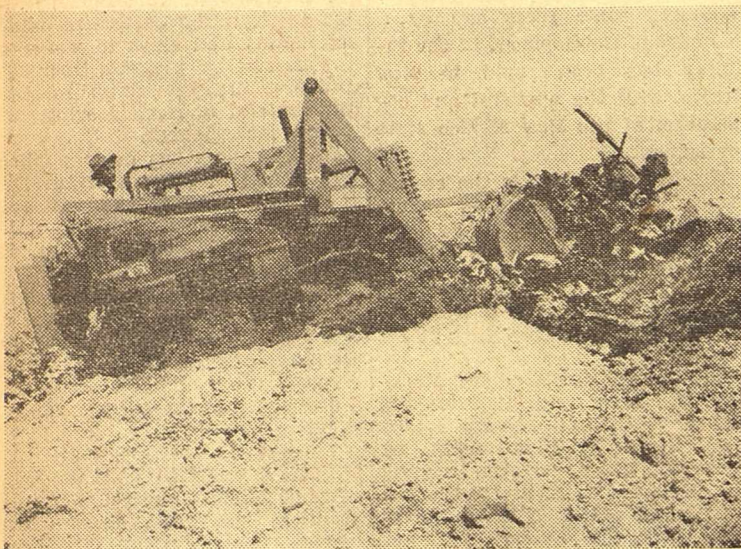
A. B. Taylor, city employe, is shown operating the Cletrac tractor which has transformed the once unsightly dumping grounds east of the city into a cleared-off tract which shows little evidence of ever being the serious health menace it was. Tons of junk were buried in long trenches dug by the tractor.
