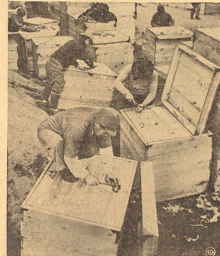
Japanese carpenters are pictured above putting the finishing touches to some of the 200 ballot boxes Tokyo will use in the national elections April 10, the first in history in which the newly enfranchised Nipponese women will take part.
