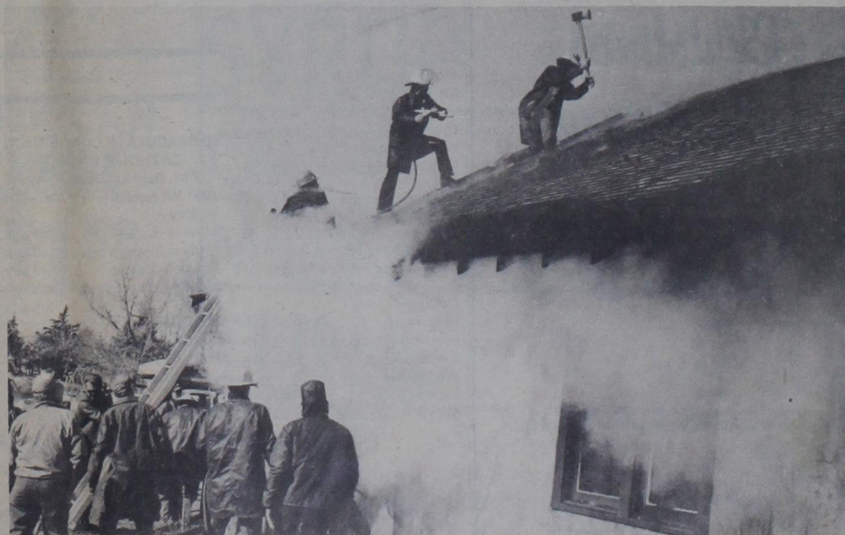
FIREMEN GO THROUGH ROOF TO FIGHT FLAMES AT LUIS GARCIA HOME Monday fire left nine persons homeless
