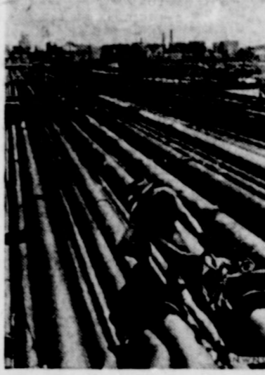
America's super-aviation fuels must be made from carefully selected crude oils. Here, at a large New York refinery, many miles of pipe lines segregate these special crude oils, which have been shipped from various U. S. oil fields, and deliver them to refinery units where 100-octane aviation gasoline is manufactured.
