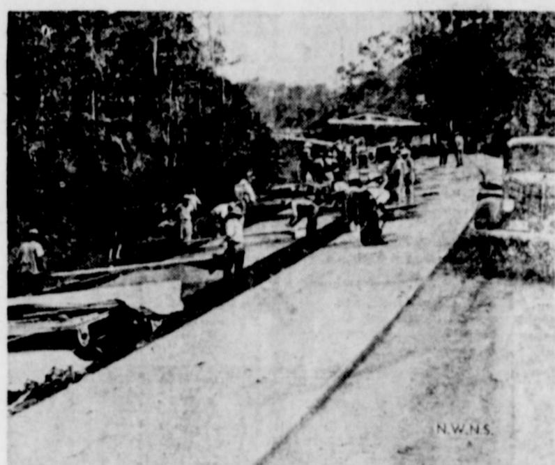
Concrete crews in the Canal Zone are shown at work on a section of the new Trans-Isthmian highway that Uncle Sam is building at top speed across the Isthmus of Panama.
