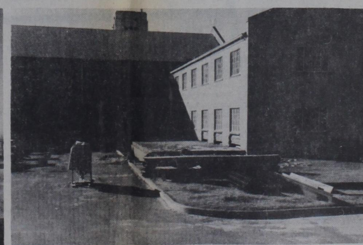
FIRST UNITED METHODIST—Work is progressing on a major remodeling project by Dimmitt's First United Methodist Church. The newly raised level alongside the north wing will soon be the floor of an enclosed foyer and separate entrance, with a new choir
