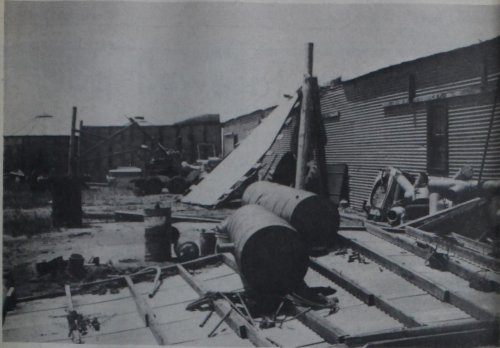
WHERE A BARN ONCE STOOD, there are now only these remnants where a small tornado struck Saturday evening on the Paul Brooks farm a mile south of Hart. In foreground is the barn's west wall, and the east wall still stands in the
