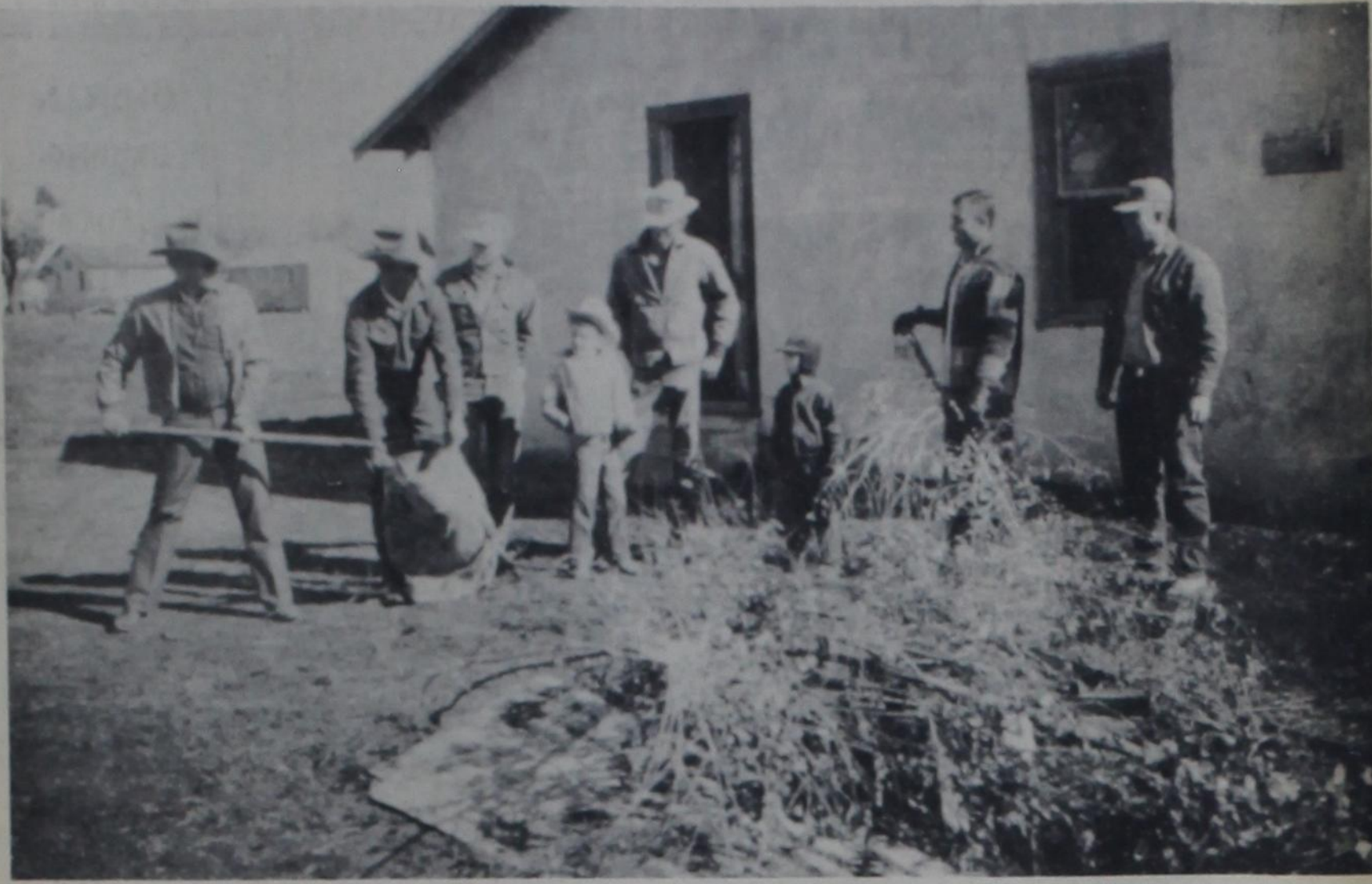
THE SCOUT HUT grounds near Dimmitt's city park got a cleaning and sprucing-up Saturday morning, courtesy of the Dimmitt Young Farmers, who cut and burned weeds around the building and made repairs to the building it-
