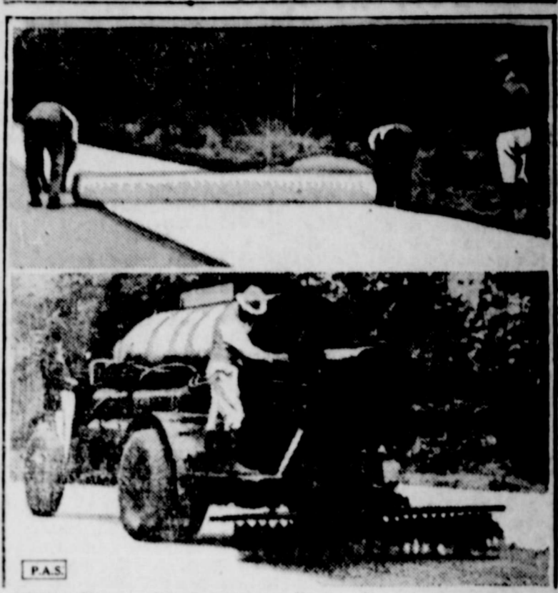
SCOTT, Miss. . . . The first "Cotton Highway", a 14-mile experiment in road construction, is rapidly nearing completion here. The upper picture shows the cotton fabric membrane being rolled out on the highway on a base of mixed clay and gravel. Lower picture shows coat of tar over cotton, this covered with two applications of asphalt mixed with screen gravel.
