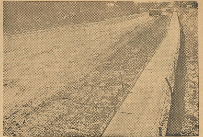
MAJOR ARTERY in local transportation is undergoing surgery for wide improvements. Front Street is presently being paved, widened and curbed to accommodate the heavy flow of traffic from the growing west part of Dimmitt. Other streets to receive improvements include E. Dulin, S. W. 3rd and 4th, E. Belsher and Halsell Streets. See story. —Staff Photo
