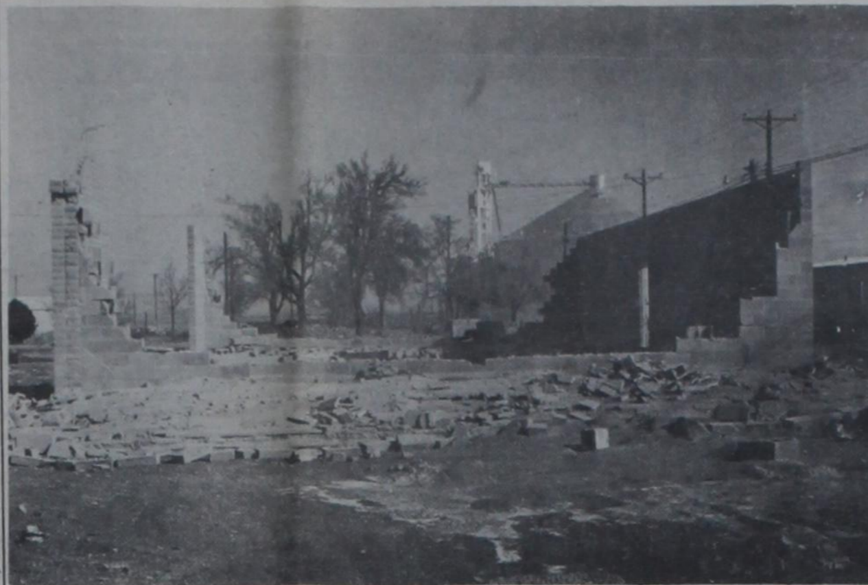
AND THE WALLS CAME TUMBLING — High winds late Wednesday night and all day Thursday brought down the north and south walls of the new Circle K store in northeast Dimmitt last week. Don Mason Builders of
