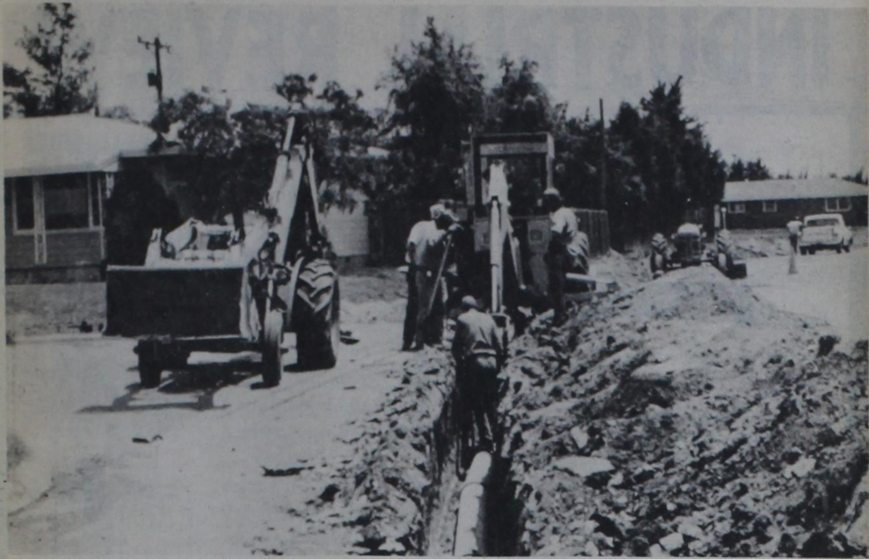
ALMOST THERE — City workmen dug up a portion of Western Circle Drive last week as they headed north toward the home stretch in the laying of water line from
