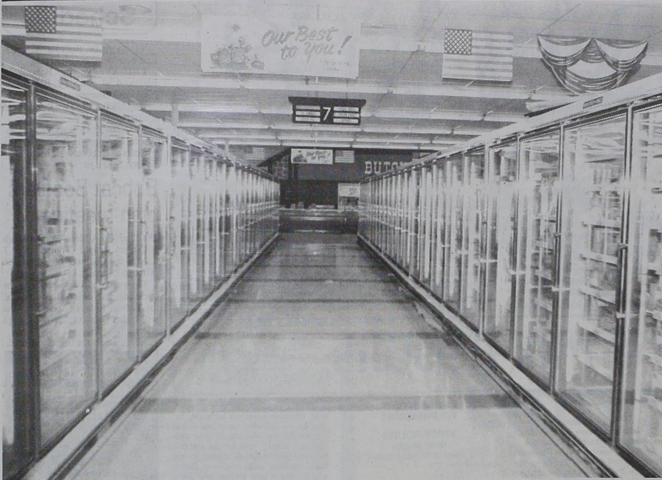
ALL NEW AND IMPROVED!—A phrase you often hear applied to products in a supermarket can now be applied to the frozen food section at Dimmitt Thriftway after installation of new upright freezer
