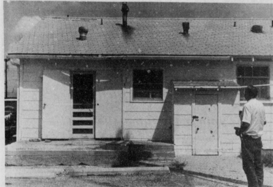
SURVEYING NEEDED REPAIRS —W. L. Thomas, Maintenance Director for the Lockney General Hospital, surveys needed repairs to the old temporary military barracks which has served as the patient rooms for the hospital since the 1940's.
