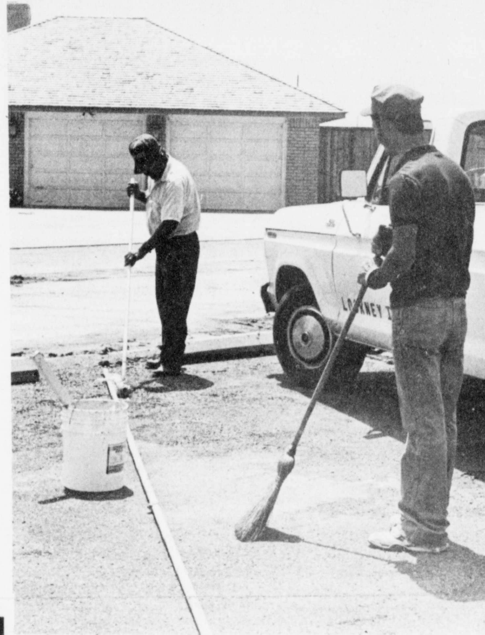
GETTING READY FOR SCHOOL-- The parking lot at the elementary school is being striped in preparation for the opening of the school year. The custodians and maintenance personnel have been busy this summer getting the schools and playgrounds ready for the influx of children. Staff Photo
