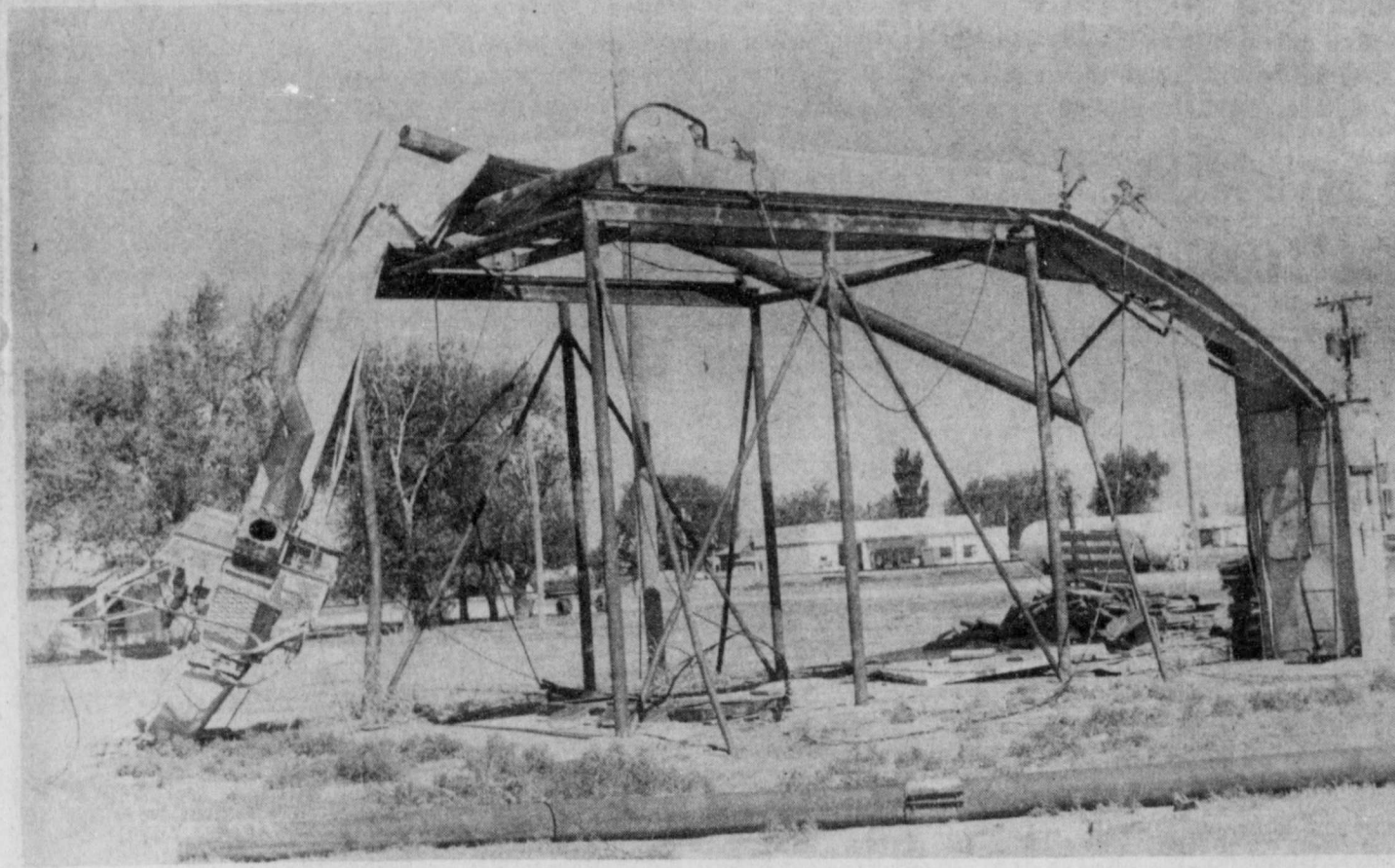
TORNADO AT SOUTH PLAINS? —The elevator leg at the Lockney Cooperatives elevator at South Plains was struck down by what appeared to be a tornado that dropped down into the community Thursday night. Dam-
