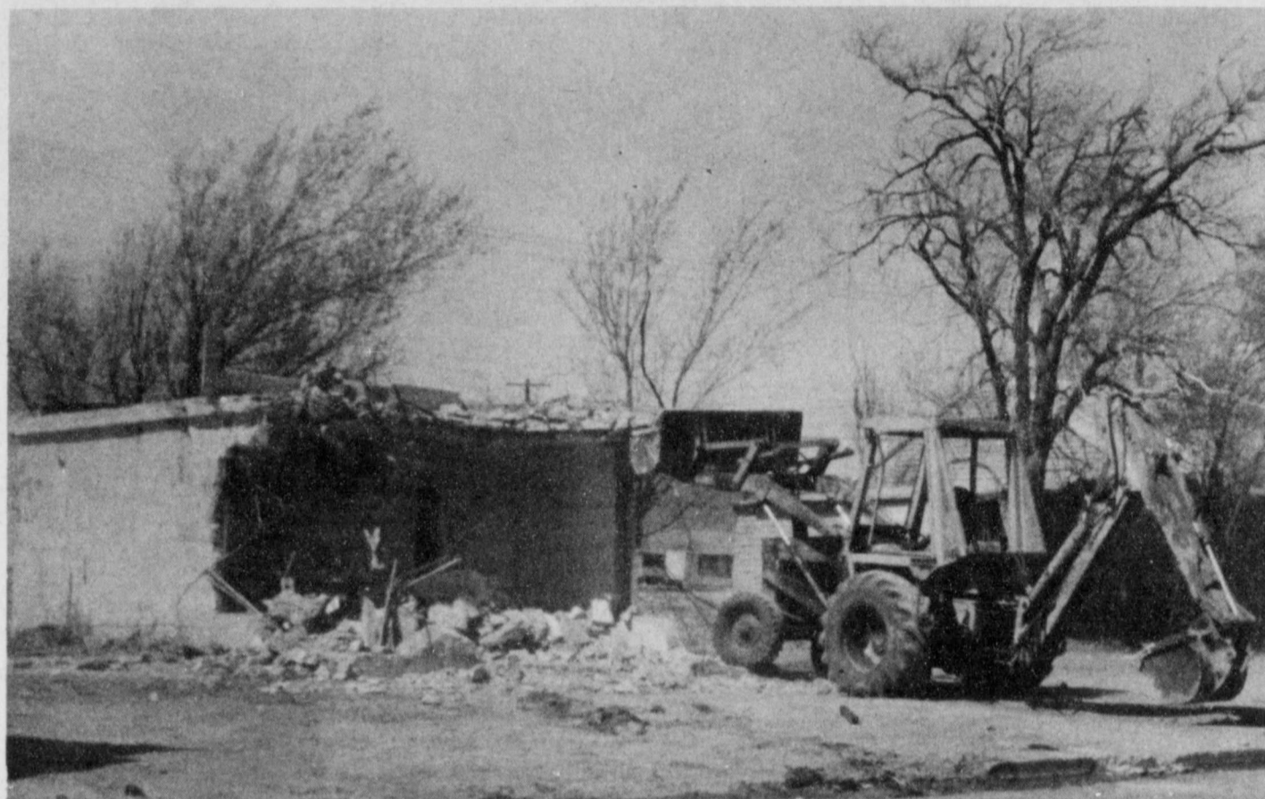
ANOTHER ONE BITES THE DUST —Another old structure in Lockney is being torn down. Last Tuesday, members of the Lockney City Council approved tearing down the old Lockney jail house, which was constructed in 1918. Following the council's approval Tuesday morning, Vernon Wickware of Floydada began tearing down the building. He was still working on the removal of the structure Tuesday of this week. —Staff photo
