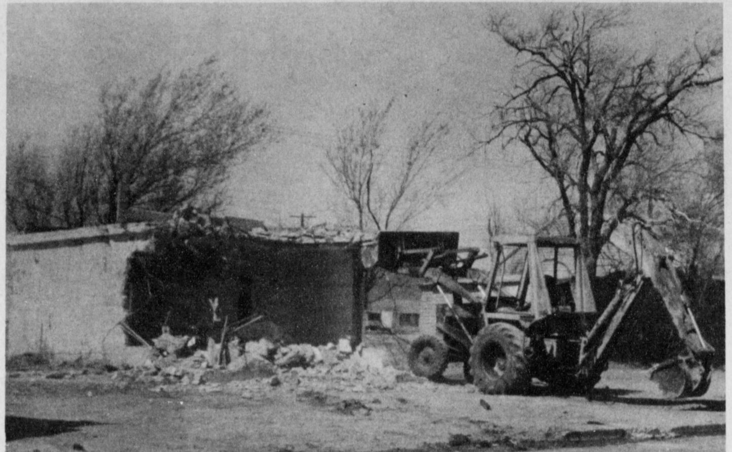
ANOTHER ONE BITES THE DUST —Another old structure in Lockney is being torn down. Last Tuesday, members of the Lockney City Council approved tearing down the old Lockney jail house, which was constructed in 1918. Following the council's approval Tuesday morning, Vernon Wickware of Floydada began tearing down the building. He was still working on the removal of the structure Tuesday of this week. —Staff photo
