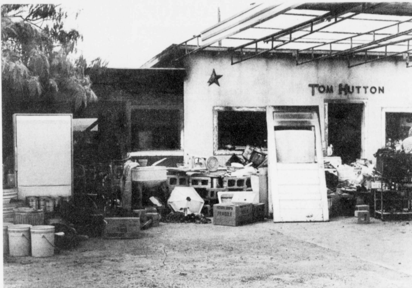
CHARRED RUINS —The Texaco service station immediately east of the Trading Post sustained extensive damage early Thursday morning. Mary Hutton, the owner, was asleep when she awakened to see a blaze in an adjacent room.
