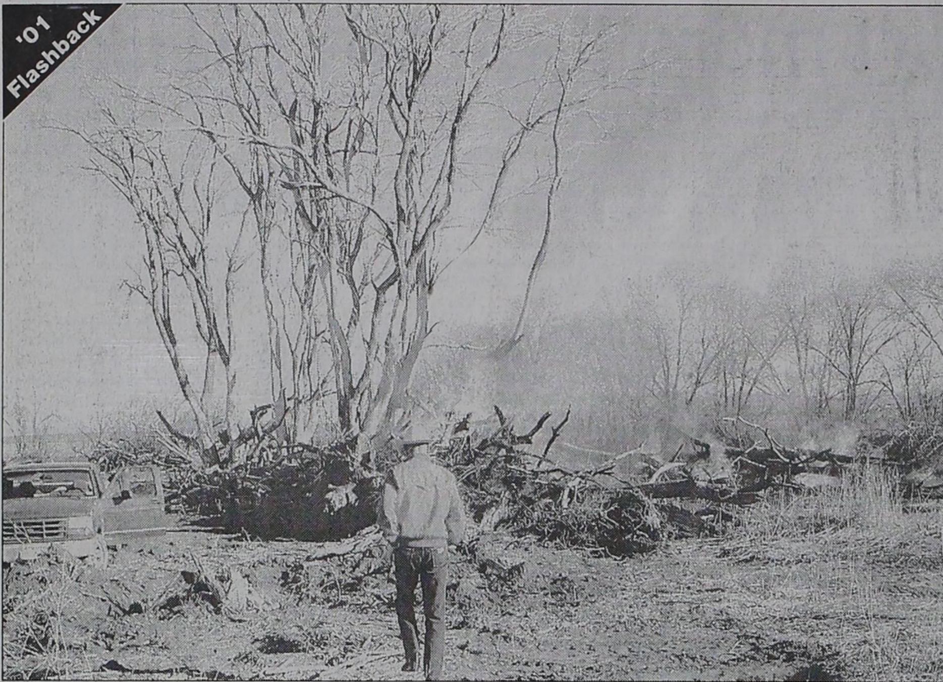
'01 Flashback THE END OF A GRIM REMINDER -Dimmitt City Manager, Don Sheffy watches as The Forest is burned and bulldozed under so that it is no longer an attraction to Castro County youth. The
