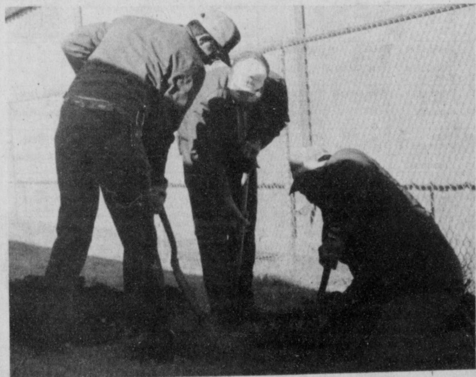
PLAYING IN THE DIRT—Employees of the city of Lockney Water Department have been seen lately digging in the dirt at various spots around Lockney. Actually the men are trying to find and correct problems with leaks and stopped up pipes. STAFF PHOTO
