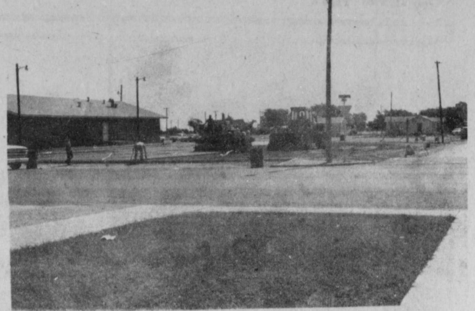
HIGH PLAINS PAVING COMPANY of Plainview completed paving the hospital parking areas on Friday.
