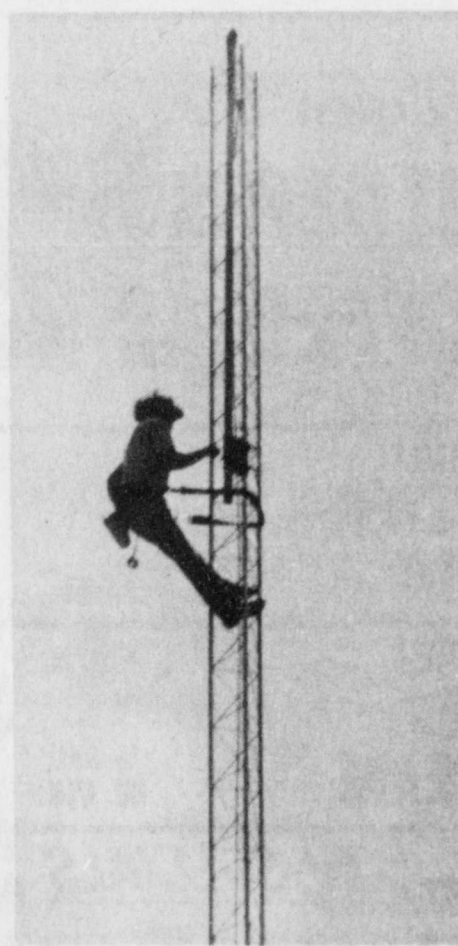
WORKMEN installed the radio tower at Lockney General Hospital Friday. The tower will enable the hospital to use a newly installed paging system for quick contact with the hospital staff members.
