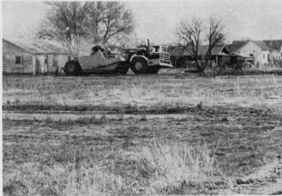
WORK CONTINUES by the Lipham Construction Company of Aspermont on the dirt roads in the northeast part of Lockney with their dirt movers and heavy road equipment.
