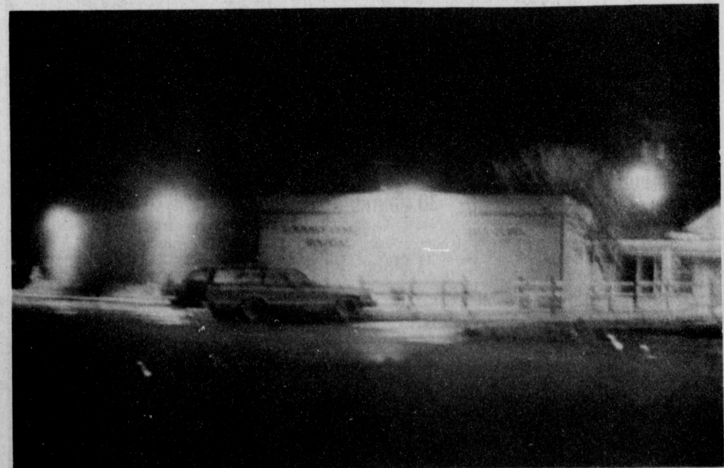
SECURITY LIGHTING was completed this week after a day or two delay because of bad weather. Pat's Electric in Plainview installed the low sodium lighting on the west and southwest corners of the clinic. The lights will be powered by an emergency generator in case of a power failure.
