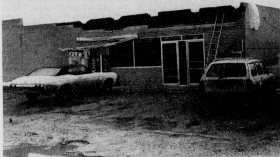
KEETER'S GROCERY suffered extensive damage to the front of the store when the weight of the snow that had collected on the awning tore several layers of brick away, exposing the roof of the building to the elements. The damage was not covered by insurance. It is feared more moisture will cause further damage.
