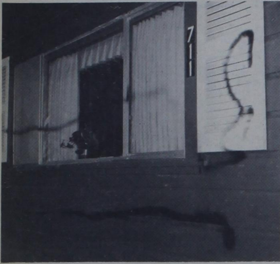
SPRAY PAINT USED ON PORCH FRONT . . . At Andy Elder home, 711 Grant St.
