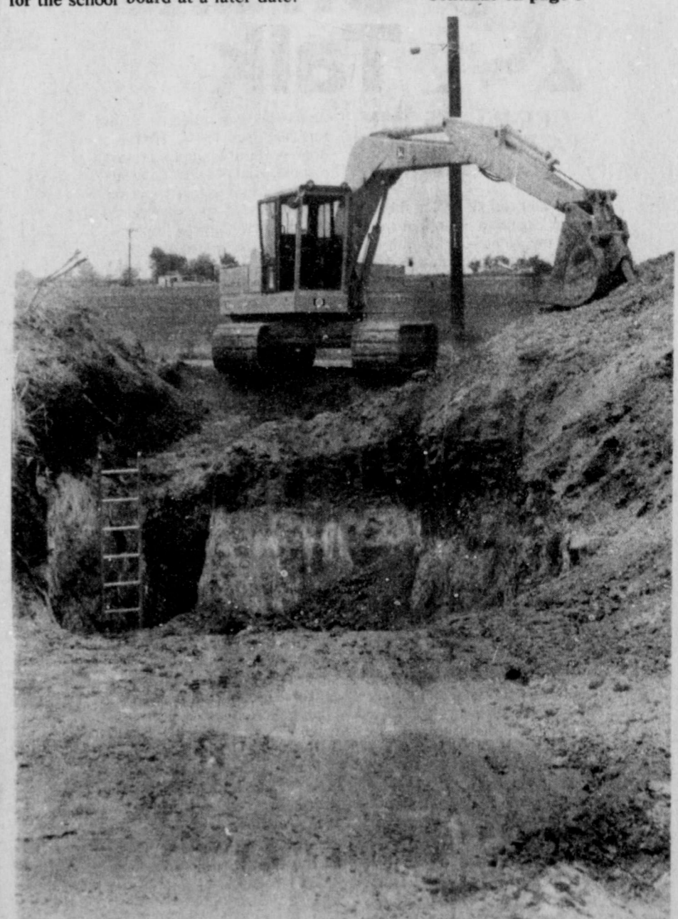
THE WORK IN THE TARGET AREA in northeast Lockney is progressing. A sewer lift will be installed on the City's right-of-way on East Guest Street. New water and sewer lines will also be installed. Paving is scheduled for early spring.
