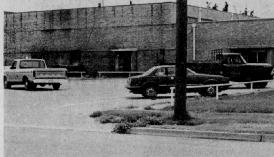
REEROOFING HAS BEEN BEGUN on the school building this week. Additional repairs and maintenance will be completed soon.
