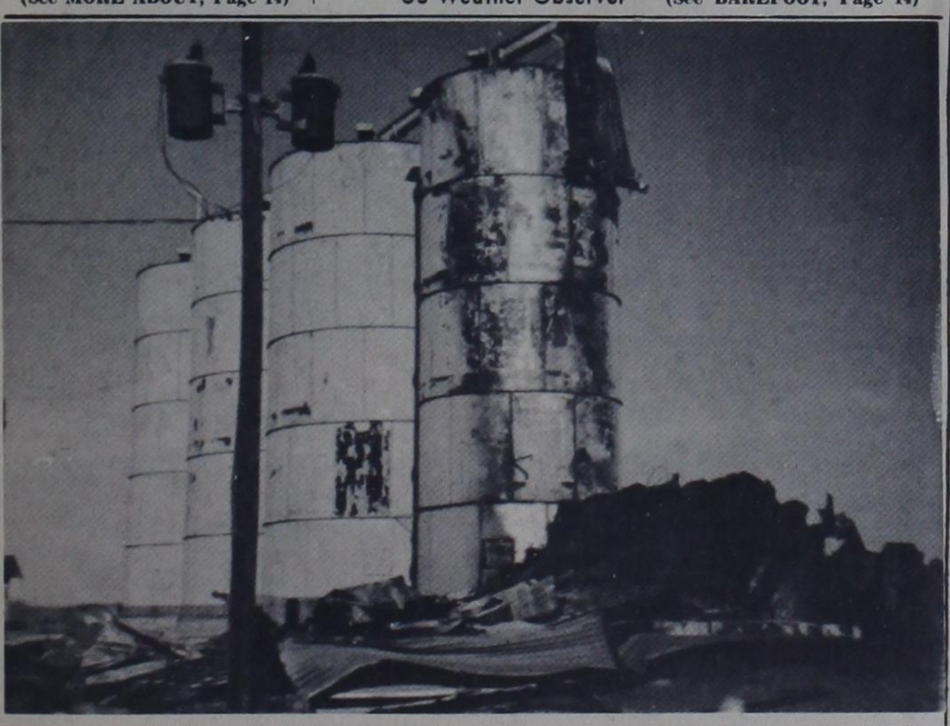
FIRE caused $10,000 to $15,000 worth of damage Saturday night to this Hart Grain Co. sub-station 7 1/2 miles east of Hart. A motorist discovered the blaze at 6:15 p.m., and firemen from Dimmitt, Hart and Edmonson fought the blaze until 8:30. Roy Burrus of Plainview, owner, said the burned portion of the elevator didn't have much grain stored in it. Cause of the fire was unknown.
