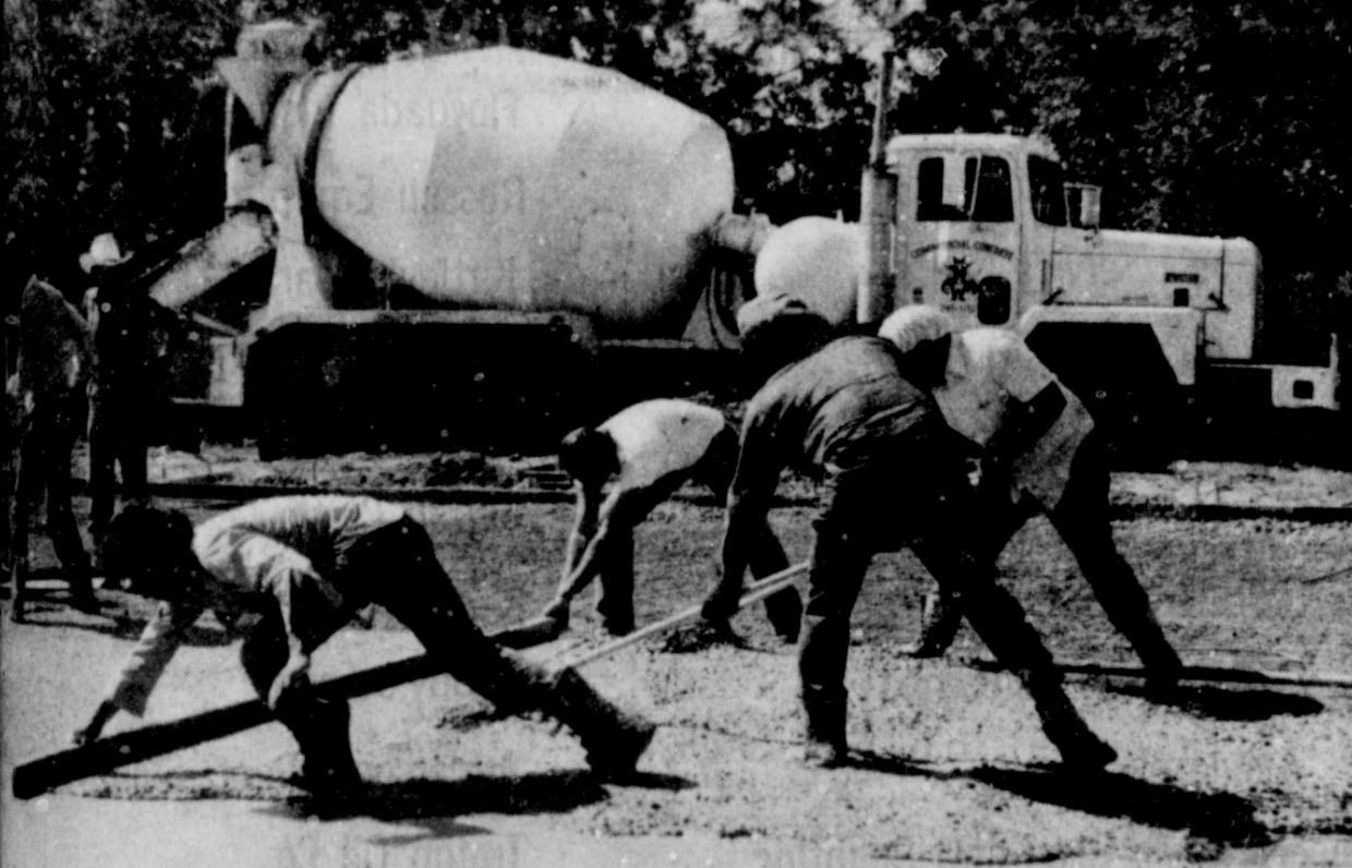
Water was poured this week for educational building at First Baptist Church in Lockney. It's expected to take about four months to complete the project.
