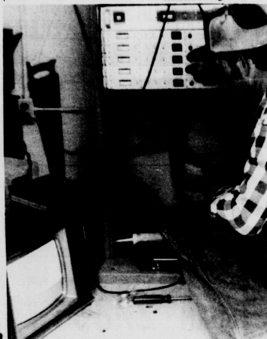
JERRY FORD OF LOCKNEY CABLE TELEVISION says pictures began coming into the systems' headquarters last weekend and it may be less than a month before the system is in operation in most of the city. Ford says he plans to begin pre-wiring houses tomorrow for cable television.
