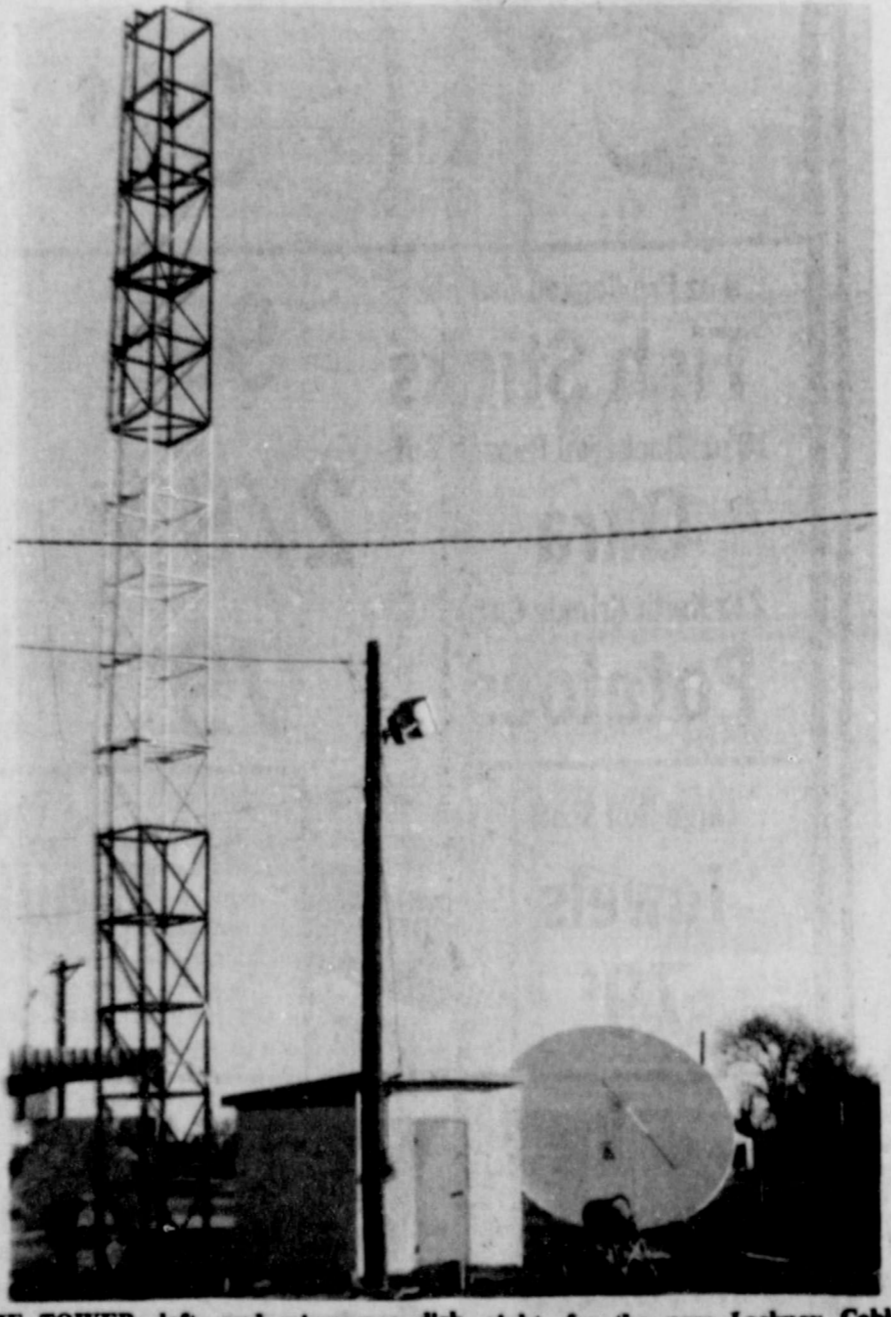
THE TOWER, left, and microwave dish, right, for the new Lockney Cable Television System have been installed. The electronic equipment for the system will be installed soon in the building at the center of the photo. System operator Jerry Ford says he hopes to have the cable working in most of the city by the end of May.
