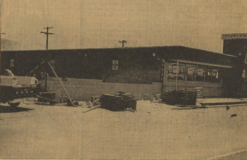
TAYLOR AND SONS GROCERY is undergoing an enlargement and remodeling program when completed, according to Macky Oldfield, store manager, will add to the convenience of customer shopping as well as to an overall improvement in efficiency operation. Work is well underway on the construction of a 40x92 foot addition to the store building. When completed the store building will be 115x92 feet. The new addition, connected to the north side of the present building, is of brick and tile and is expected to be completed six to eight weeks. Present plans are to remodel the entire building and to add a considerable amount of new equipment and fixtures. The store property will provide 30 feet of parking space on the north side of the store for employee parking, while the present customer parking area on the south side of the building will be scribbled for more efficient parking. Taylor and Sons have been operating the store since purchasing the Cashway Grocery from Wimpy Walker three years ago. G. L. Willis is owner of the building.
